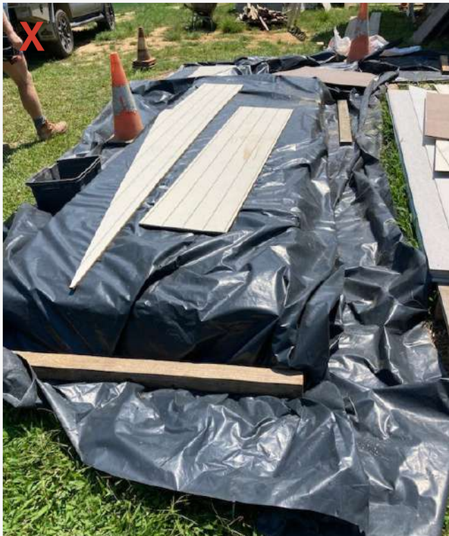
Incorrect storage of Easycraft products, stored outside and wrapped in plastic
