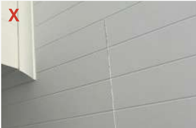
Panel joints showing when panels are installed end to end with no expansion gap or decorative trim cover
